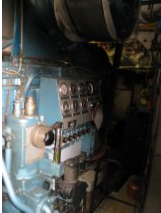
Engine control panel
